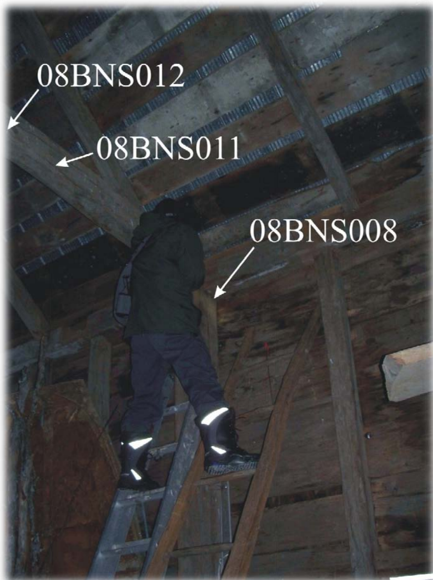
Figure 6. Sample 08BNS008 being taken from a large vertical beam in the barn. Samples 08BNS011 and 08BNS12 were taken from the large horizontal beam above 08BNS008.
